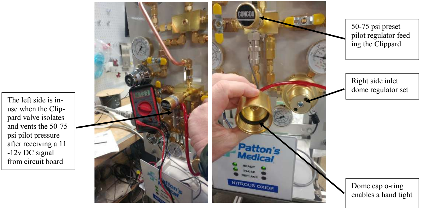
Figure 9. Showing vent tube disconnected from valve and right side inlet regulator dome cap removed.
