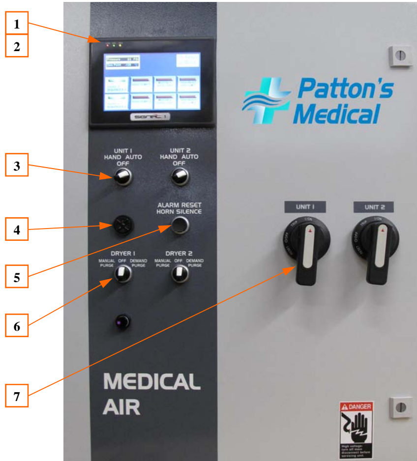
Duplex Control Panel
