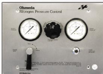
Ohmeda Gas Control Panel
